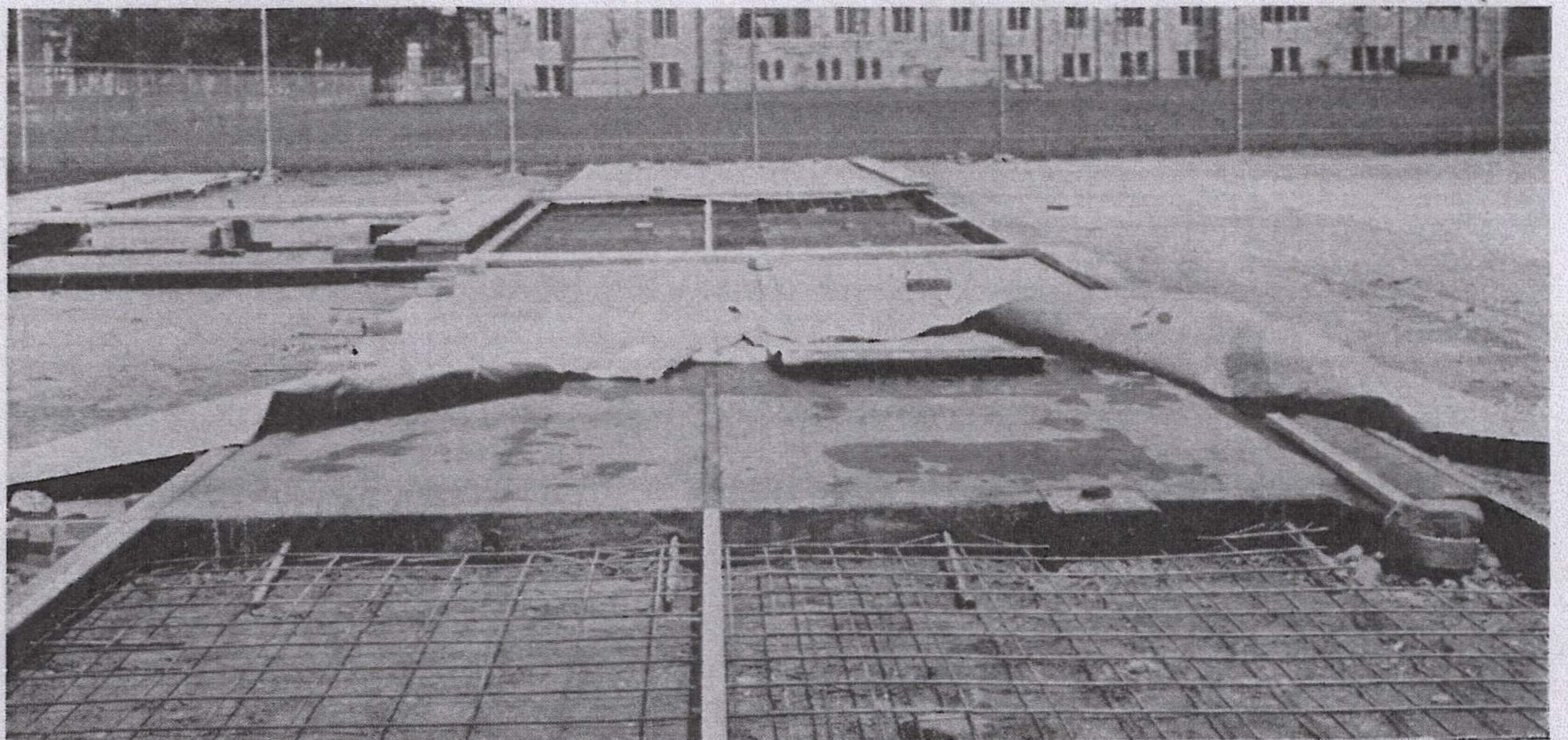
Construction view showing strips that form grooves for playing lines; reinforcement; dowels; gutter, which carries surface water to drain; base for net posts separated by tarred expansion joints. Waterproof paper used in curing is turned back to show that concrete is moist.
