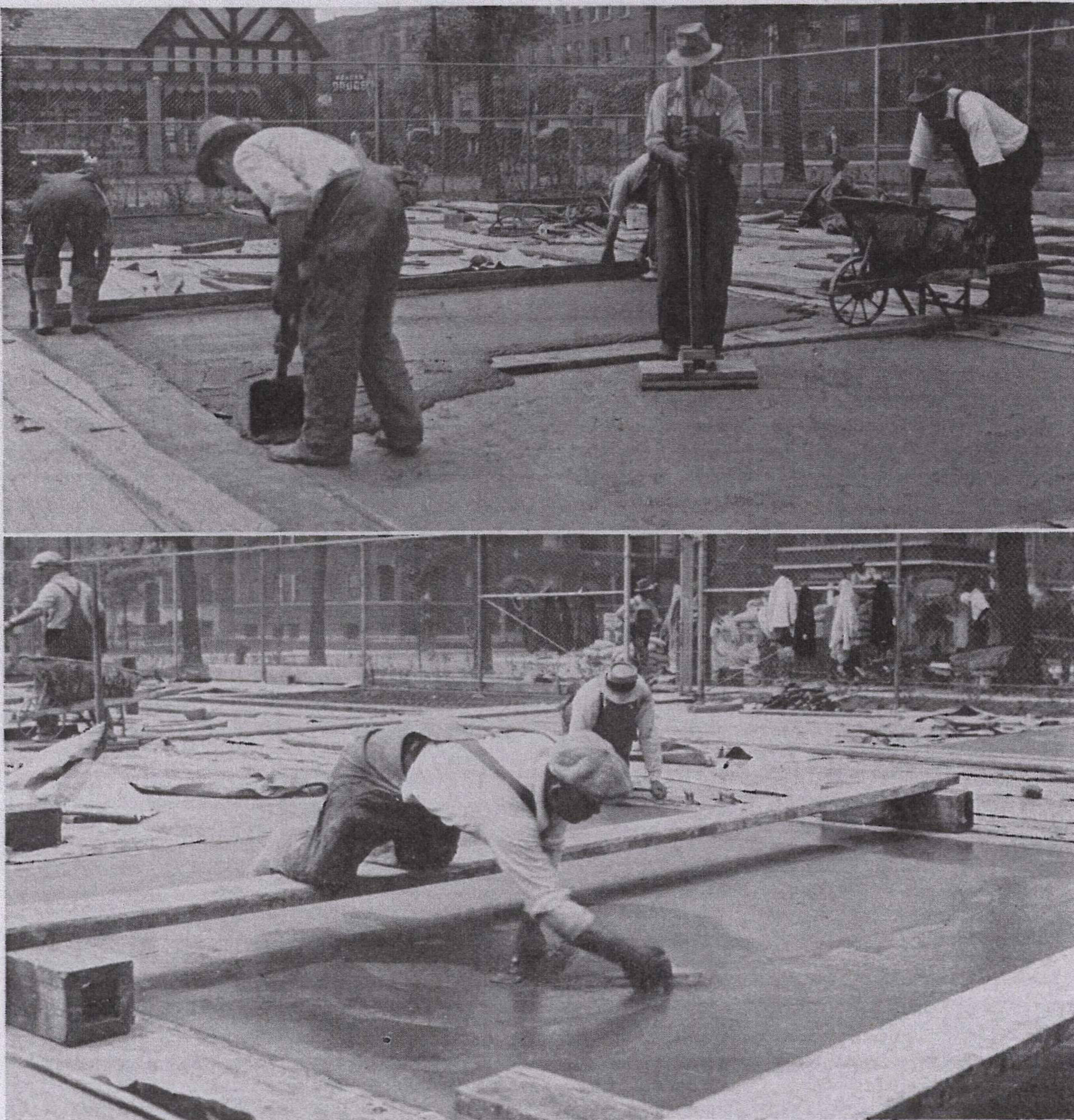
Colored topping being placed over concrete base which is tamped to compact it. Fairly stiff concrete used in both base and top. (Below) Finisher doing rough steel-troweling immediately after topping has been floated.
